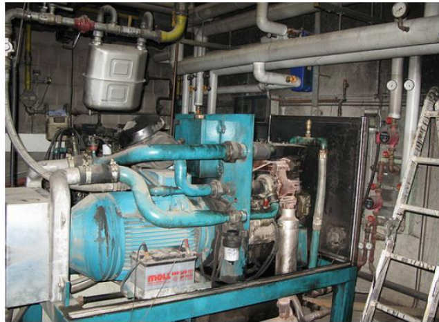
Fig 3. Combined heat and power (CHP) unit [7].
