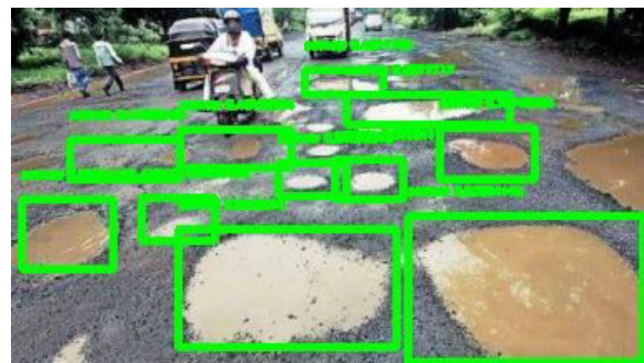
Fig 2 Potholes Detected Image
